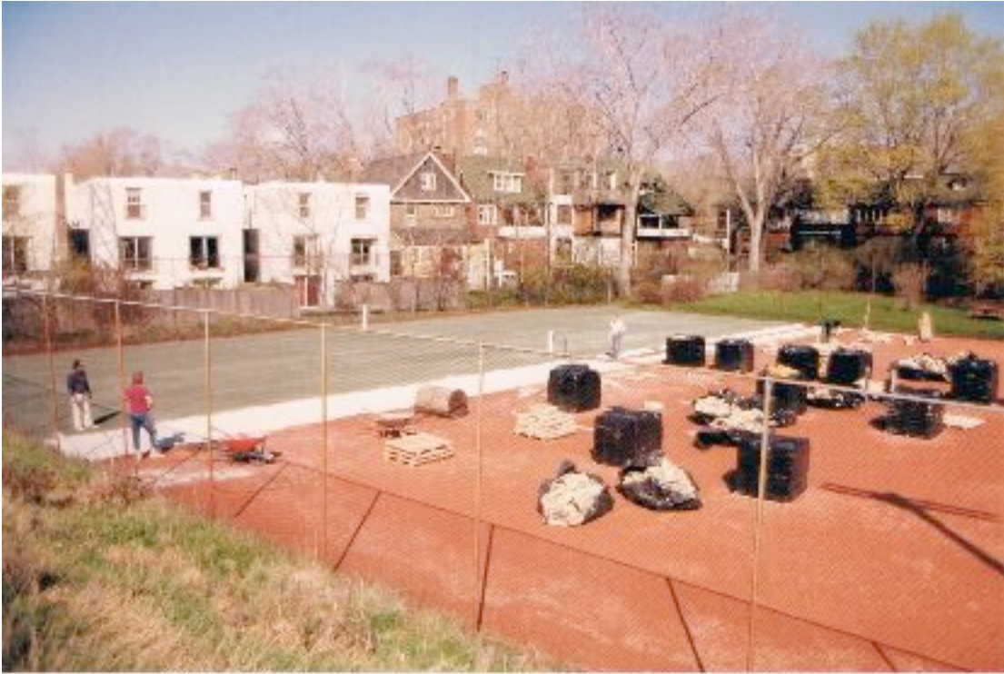
Laying the new surface on top of the old red clay. Note the brand new town houses under construction on Sydney St. to the left. (Photos courtesy Pam Portanier)
